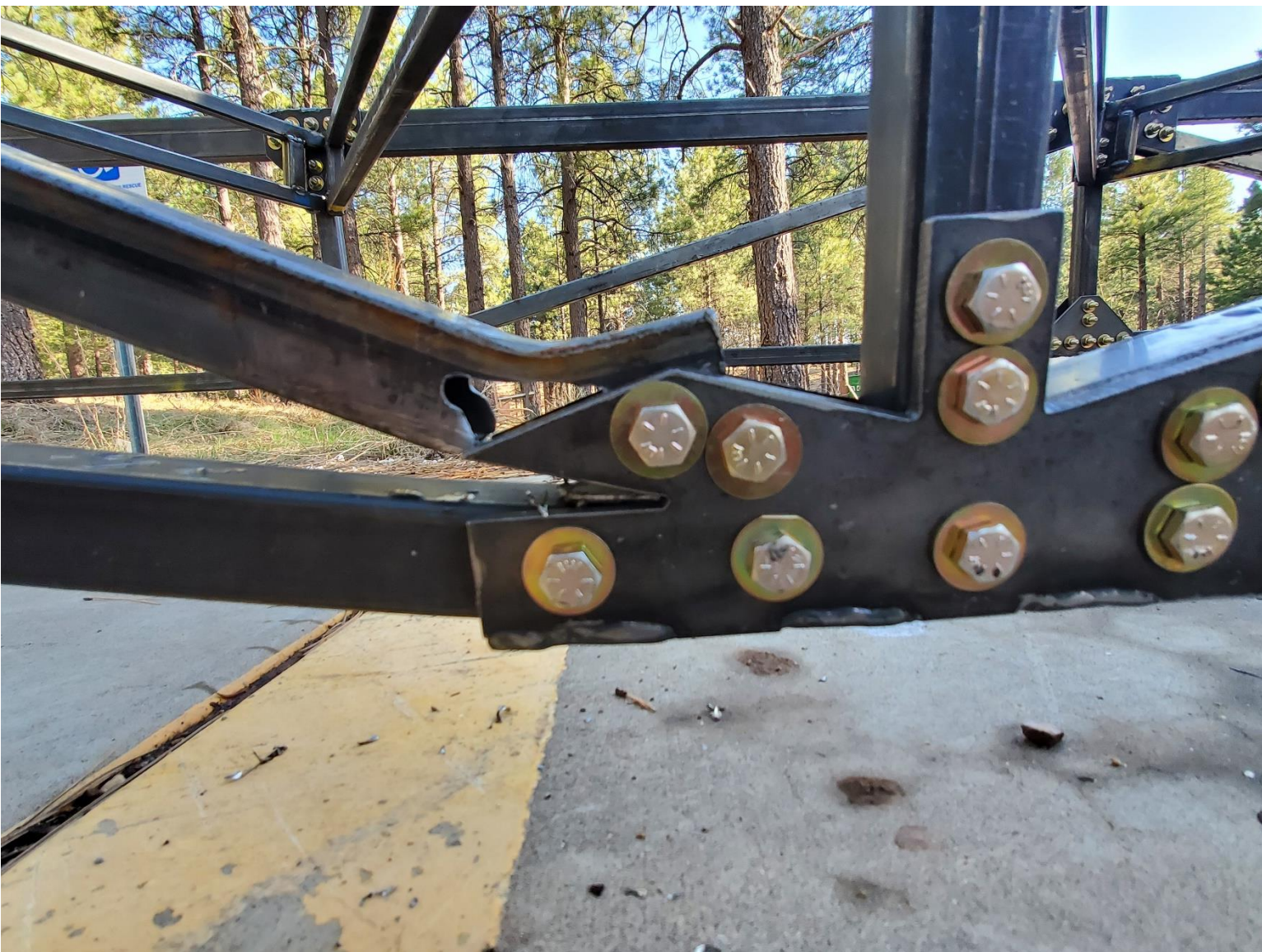
Figure 6: Member failure from loading.
